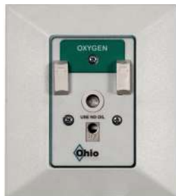
Chemetron Compatible Wall Outlet
